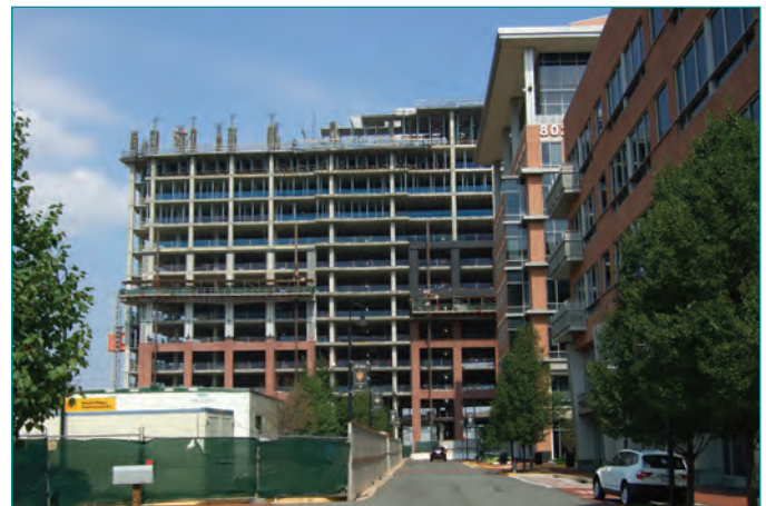
1850 Towers Crescent in Tysons Corner is scheduled to deliver 295,000 square feet of office space in April 2009.
