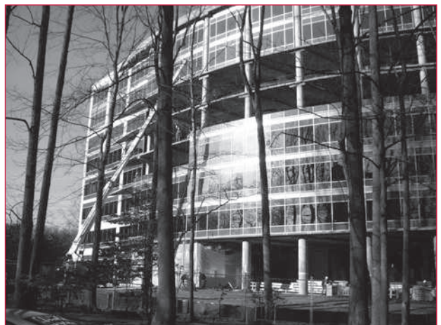
The newest office development in Fairview Park (Merrifield) is 3120 Fairview Park Drive—184,000 square feet scheduled for June 2008 delivery.
